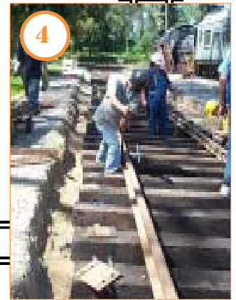
4 April 9: Rails are laid out, bolted together and spiked down by volunteers.
