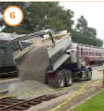
6 Mid-April: Ballast is delivered directly to the job site by "truck & transfer" at 25 tons per load.
