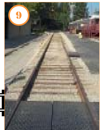
9 August 1: The completed Track 5-West is now ready and waiting for its cadre of historic locomotives and cars to be moved into display position.
