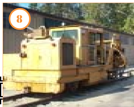
8 July: A crew from Sharp & Fellows Co. machine-tamps the ballast and surfaces the track, bringing it to the final level and alignment. The large yellow machine does the tamping; the rest of the work is done by hand.
