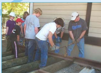
Setting one of the 1860s "55-pound" rails into place on the log ties. To the extreme right is the modern "136-pound" rail of today - look at the difference!
